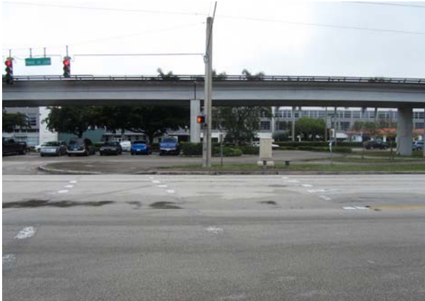
1. INTERSECTION REDESIGN The crosswalk across Ponce from San Amaro to the M-Path is very faded.
