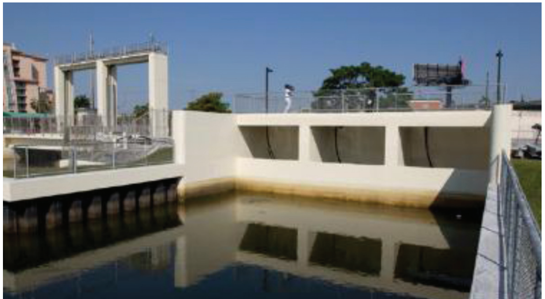
Figure 18: Forward-pumping stormwater structure. Photo courtesy of South Florida Water Management District.
